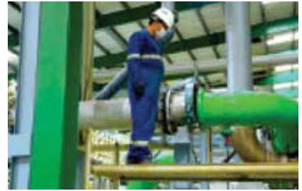
SEWA Distribution Line, UAE
