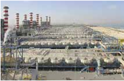
Maintenance Jebel Ali Power Plant, UAE
