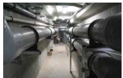
Data Center Eindhoven, Netherlands
